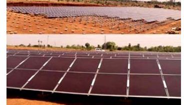
Capacity: 1MW Type: Ground Mounted Location: Bolangir India
