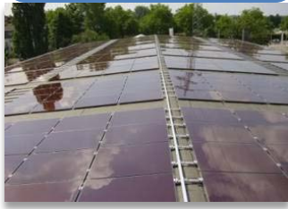
Commercial Rooftop PV system
