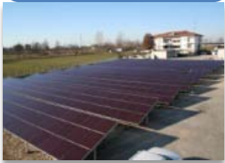
Ground mounted PV system
