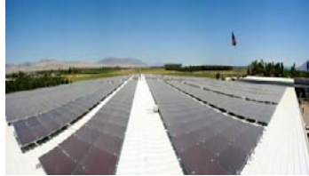
Capacity: 285KW Type: Rooftop Location: California America
