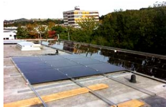
Capacity: 92.16KW Type: Rooftop Location: Dusseldorf, Germany
